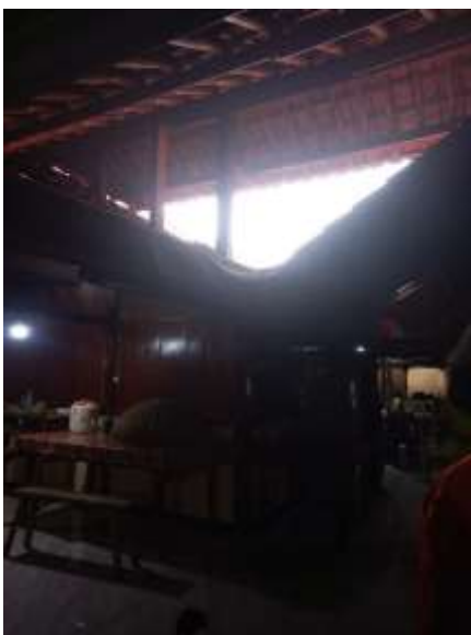
Picture 8 air holes House of Mr Supriyadi
